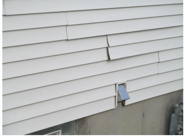
Loose siding and deterioration at vinyl siding of Building 32
