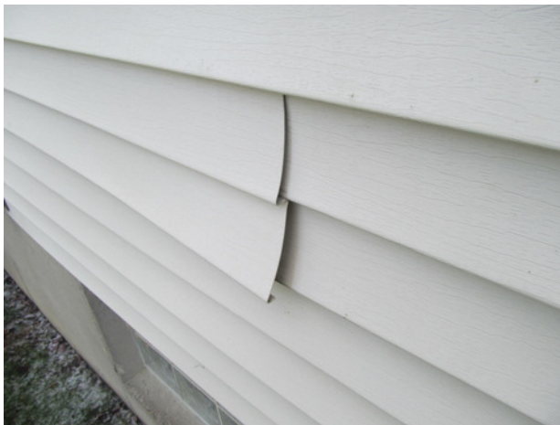
Loose siding and deterioration at vinyl siding of Building 4
