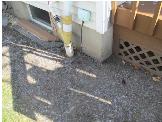
Broken, damaged and deterioration downspout connector at 32 Southwick Drive
