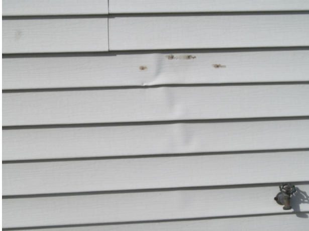
Warping and deterioration at vinyl siding of Building 19
