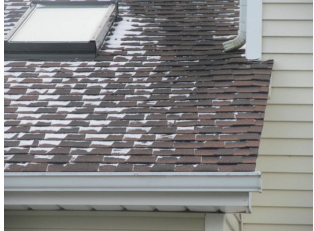
Shingle lift, stains and deterioration at asphalt shingle roof of Building 12
