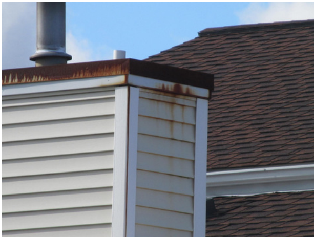
Stains and deterioration at vinyl siding of Building 30 due to chimney cap rust
