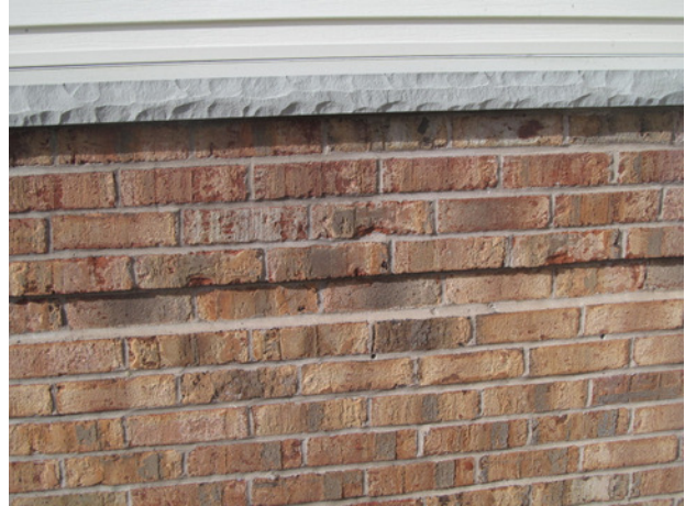
Isolated area of minor spalling at masonry wall of Building 2
