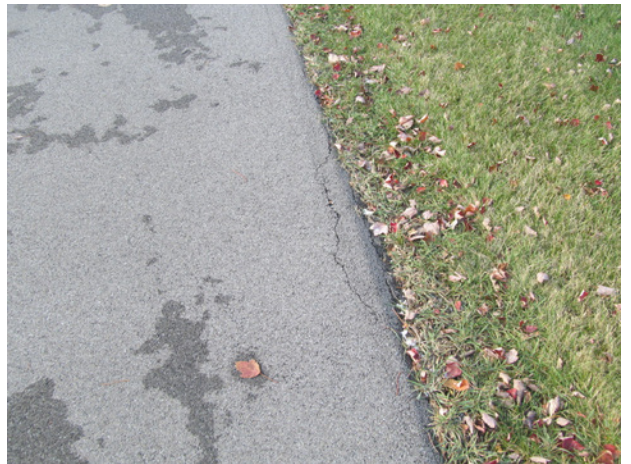
Edge cracks and deterioration at asphalt driveway of 146 Southwick Drive
