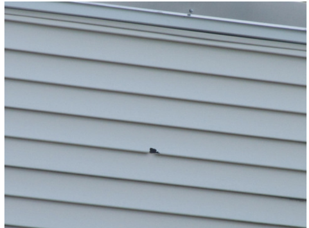
Damage and deterioration at vinyl siding of Building 24
