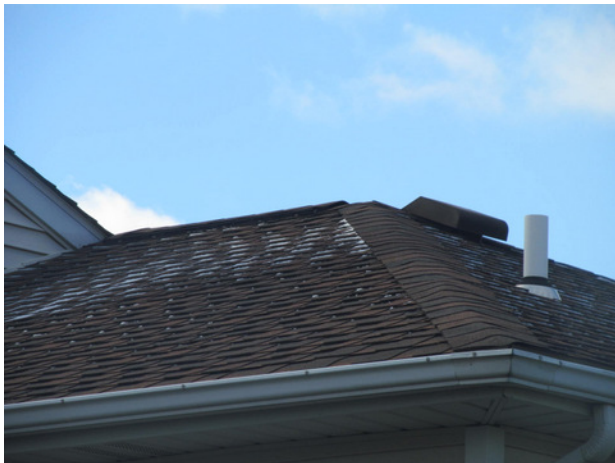
Typical ridge and square hood box hood vents, and typical rubber seal with metal base boot flashing at waste pipe penetration at asphalt shingle roof
