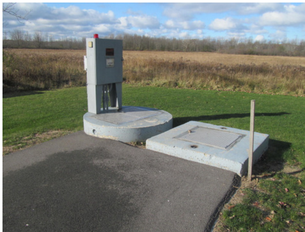
Lift station overview
