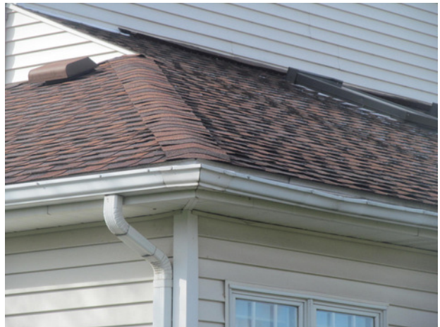
Shingle lift and deterioration at asphalt shingle roof of Building 22
