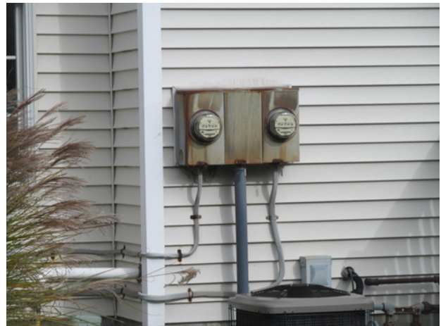
Rust and deterioration at electrical meters and panel of Building 15
