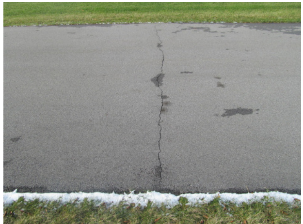
Lateral cracks and deterioration at asphalt access drive near of 130 Southwick Drive
