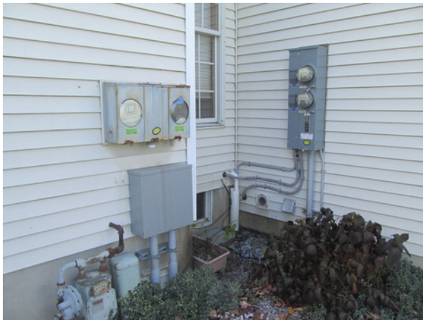
Recently replaced electrical panels and meters at Building 27 (note the Association should remove original, abandoned meters and panel)
