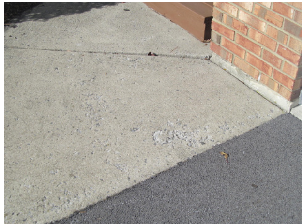
Isolated spalling and deterioration at concrete sidewalk near 26 Crabapple Court
