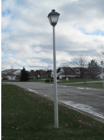
Typical light pole and fixture
