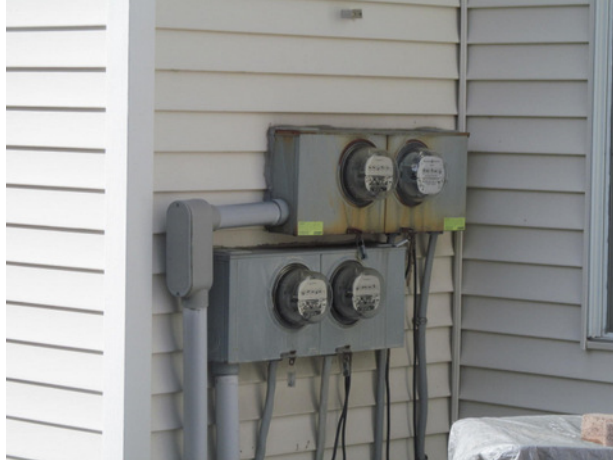
Rust and deterioration at electrical meters and panel of Building 27
