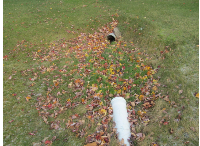
Silt and soil buildup evident at drainage culverts near Building 22
