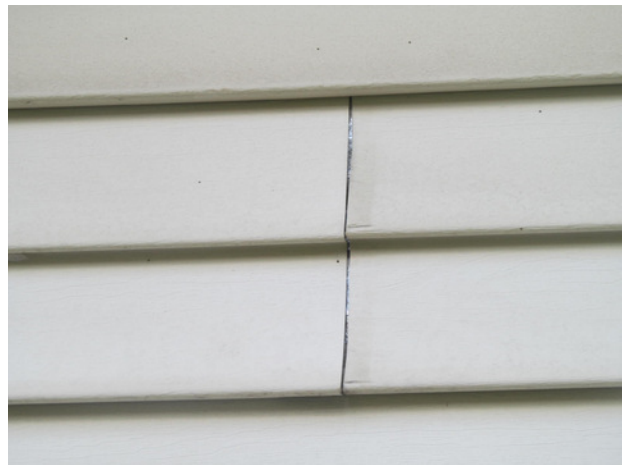
Gaps and deterioration at vinyl siding of Building 1
