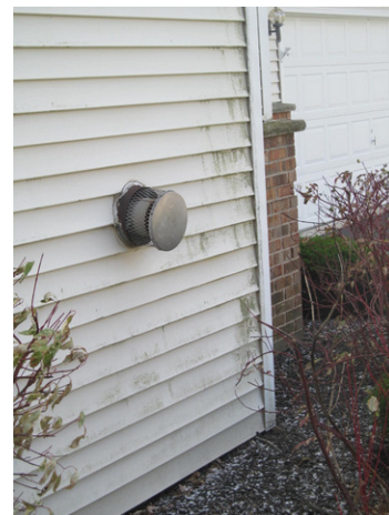
Organic stains and deterioration at vinyl siding of Building 20
