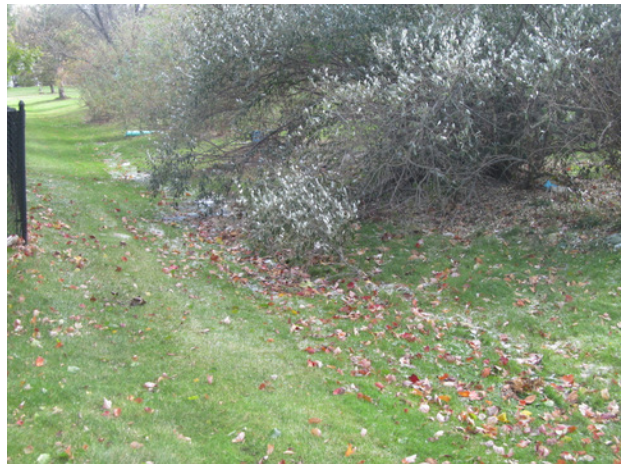
Tree branch obstruction at drainage swale near Building 1
