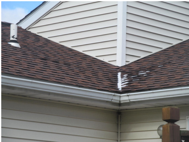
Shingle lift and deterioration at asphalt shingle roof of Building 15
