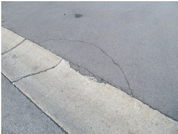
Edge cracks and deterioration at asphalt access drive near Building 6
