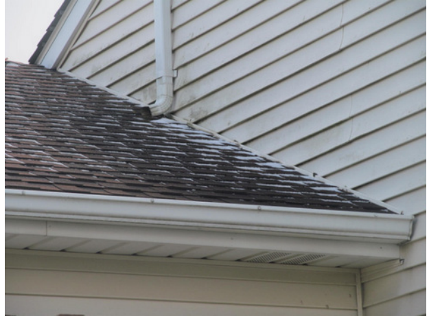
Typical downspout discharge directly onto lower asphalt shingle roof
