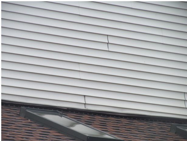
Gaps and deterioration at vinyl siding of Building 17
