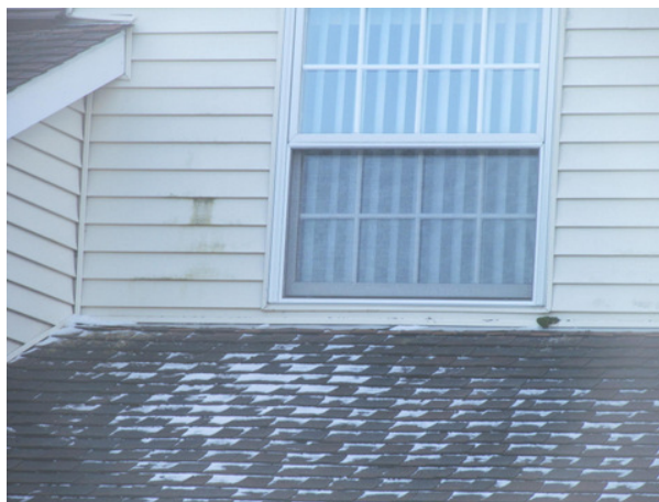
Stains, organic growth and deterioration at vinyl siding of 146 Southwick Drive
