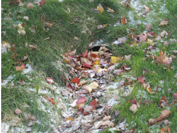
Silt and soil buildup evident at drainage culvert near Building 1
