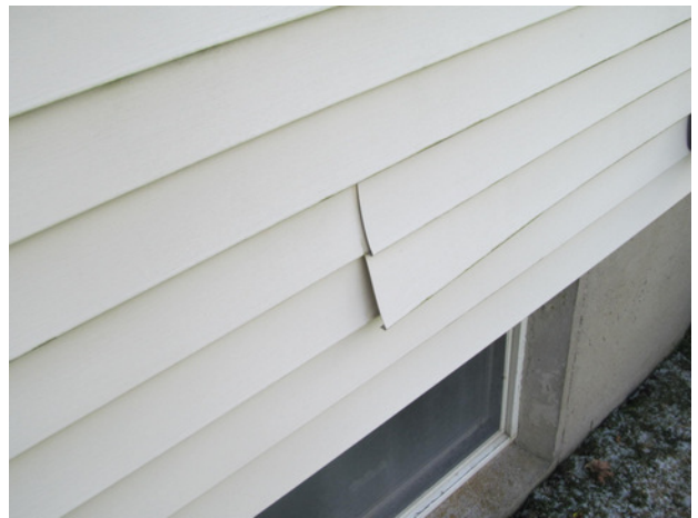
Loose siding and deterioration at vinyl siding of Building 10
