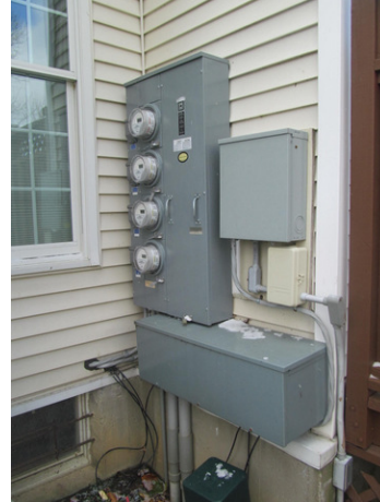
Recently replaced electrical panels and meters (note good condition)
