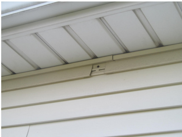
Gaps and deterioration at vinyl siding of Building 15
