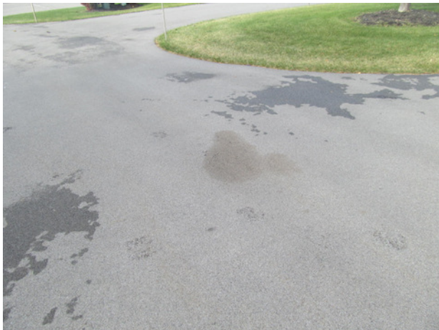
Isolated vehicle fluid stain and deterioration at asphalt driveway of 130 Southwick Drive
