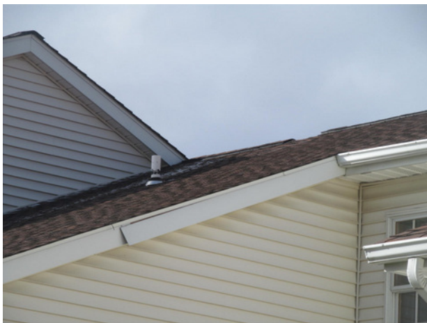
Loose cladding and deterioration at fascia of Building 20
