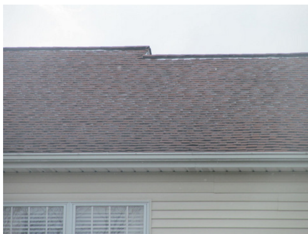
Shingle lift and deterioration at asphalt shingle roof of Building 5
