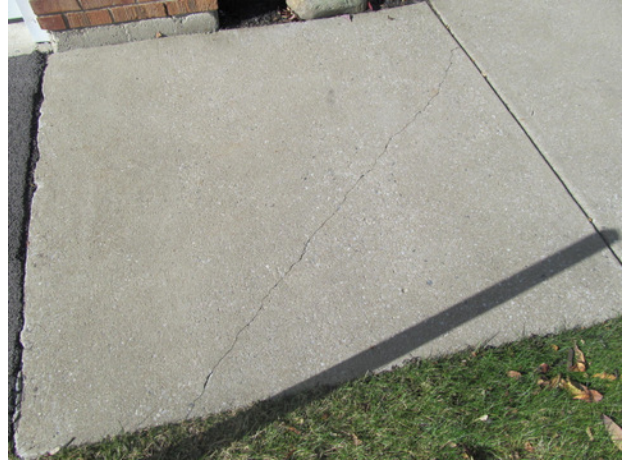
Localized crack and deterioration at concrete sidewalk near Building 25
