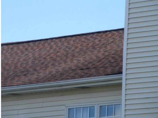
Shingle lift and deterioration at asphalt shingle roof of Building 26
