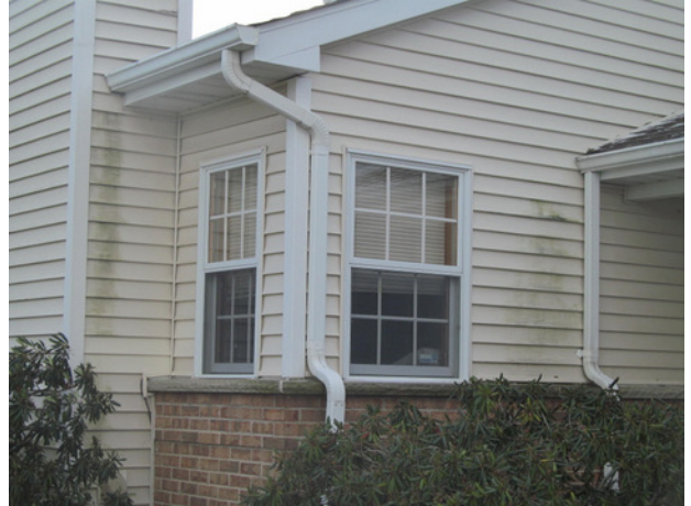
Organic stains and deterioration at vinyl siding of Building 18
