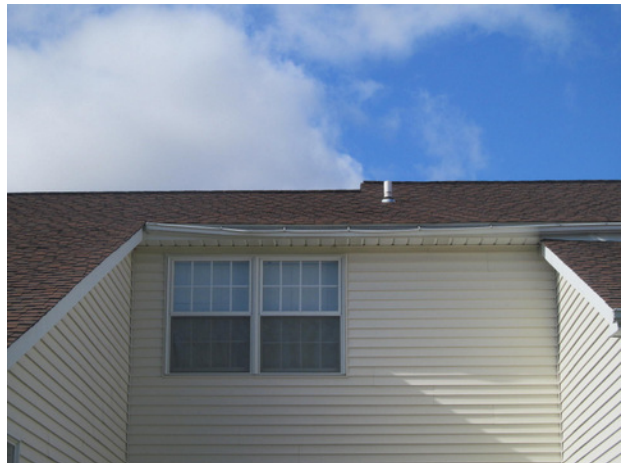
Displaced and deteriorated aluminum gutter at Building 37
