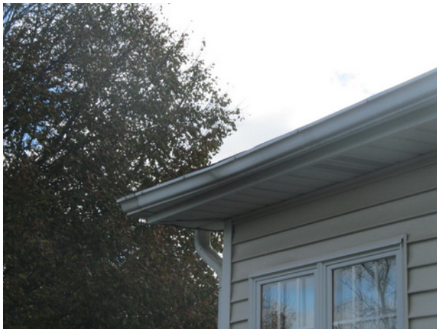
Displaced and deteriorated aluminum gutter at Building 18
