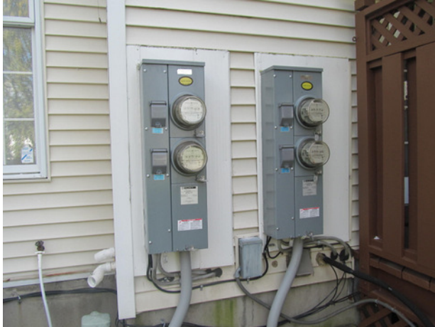
Recently replaced electrical panels and meters (note good condition)
