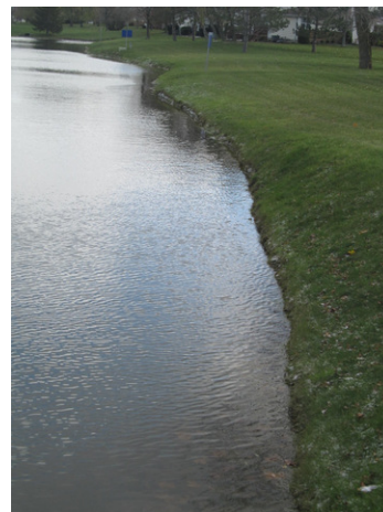
Localized shoreline erosion and deterioration along west portion of pond shoreline
