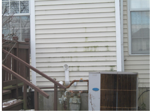
Organic stains and deterioration at Building 6
