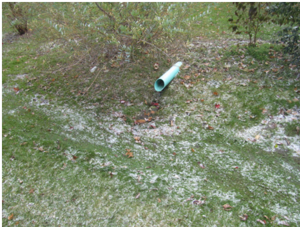
Minor erosion and deterioration at wall of drainage swale near Building 1
